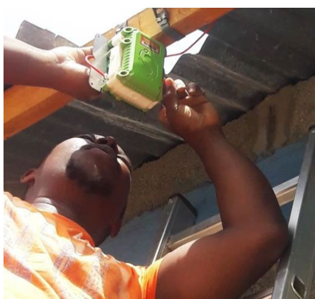
Sensors, like the one being installed at this borehole well site in Afar, Ethiopia, are helping provide key water data to address critical water supply challenges.
